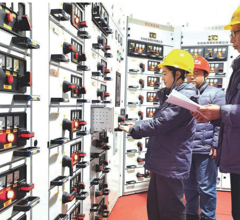
"Black Launch" emergency drill carried out by Hubei Enshi Hydropower Company
