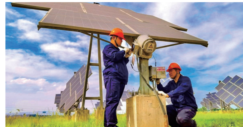
Workers of Guodian Power Ningxia New Energy were adjusting and maintaining the cell panel servo system
