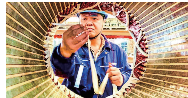
An electrician from the electrical repair workshop of Shendong Coal was engaged in motor wiring operations
