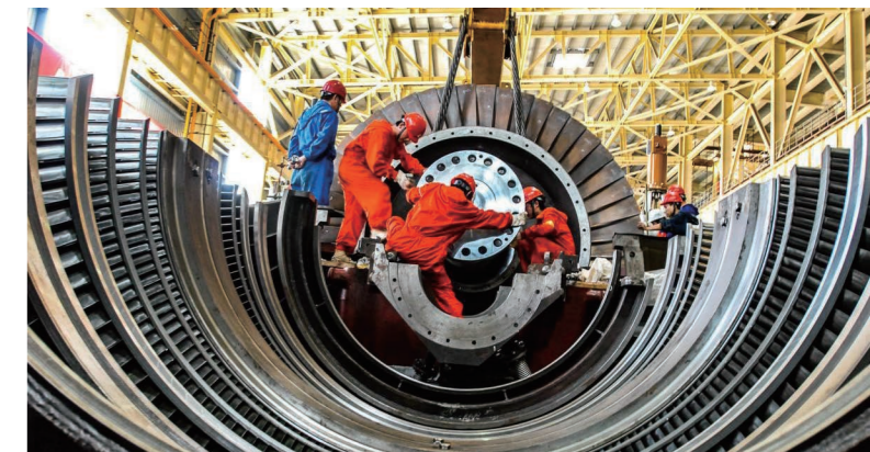
Production workers of Zhejiang Company’s Beilun Power Plant were carrying out turbine blade overhaul
